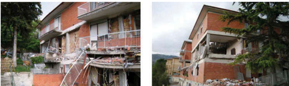
Figure 2. Second story collapse of a residential RC frame building in L'Aquila [Augenti and Parisi, 2010].
