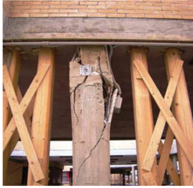
Figure 1. Column shear failure at San Salvatore hospital in L'Aquila [Augenti and Parisi, 2010].
